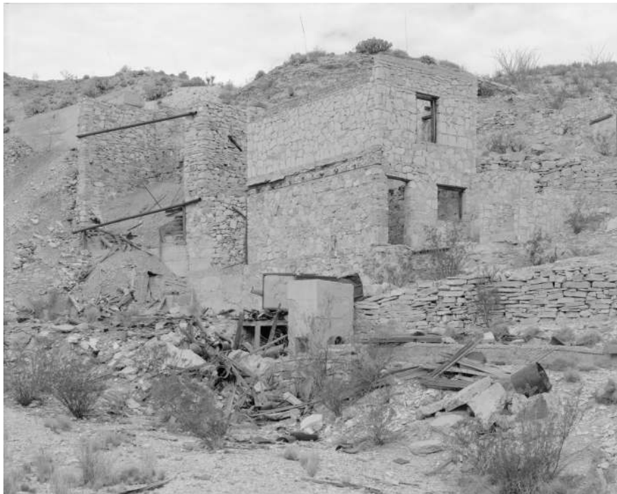
The top floor and the roof are missing in this view of the office structure. Firebricks were mixed with stone from the site to build the first floor, while firebrick alone was used to form slots for the floor joists (middle of image) and roof joists (top). Photo by Bruce Harms.
