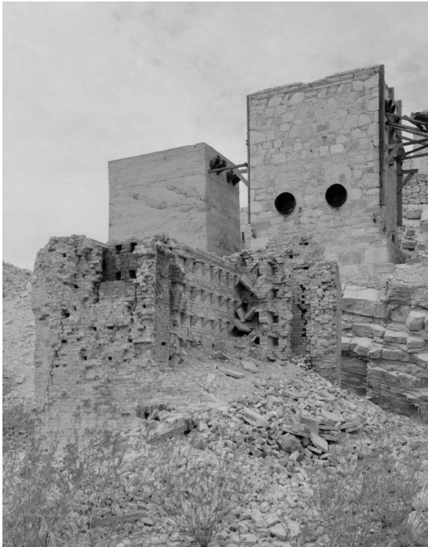
The ruins of the Mariscal Scott furnace (foreground) are only one-third the height of the complete furnace. Behind the furnace are two of the three mercury condensers. HAER photo by Bruce Harms.
