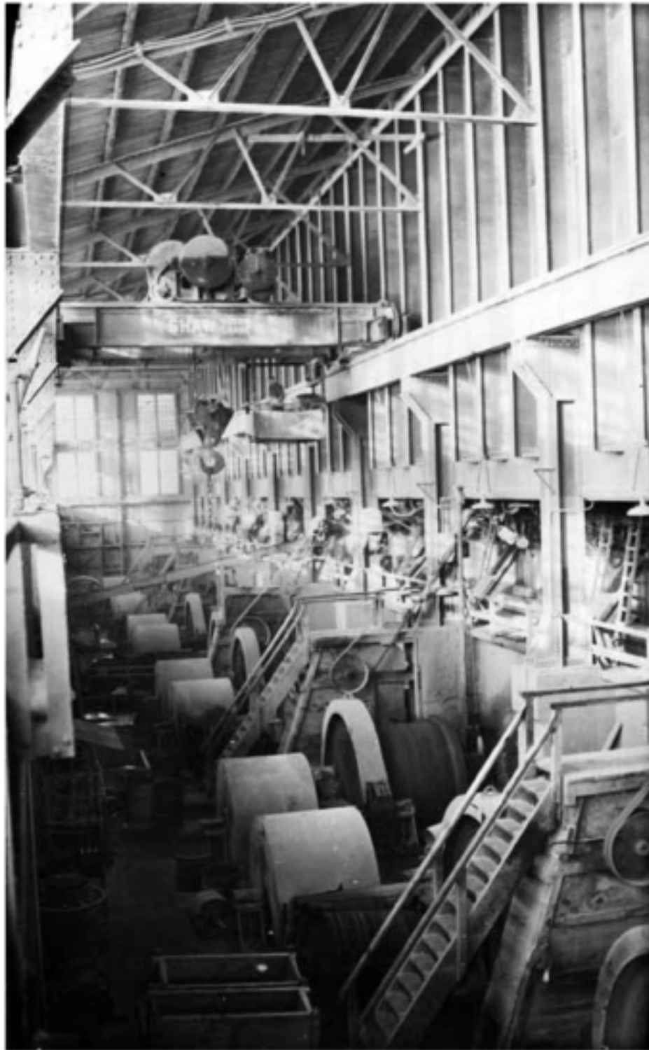
Figure 9. The ball-mill floor at the Alaska Juneau Mill, scene of a fatal accident in 1928. Note the traveling crane and operator at mid-distance, and safety guards covering the ball mill gearing. Note also boxes and equipment on the floor and the steep pitch of stairways and access ladders. (Alaska State Library Place File Photographs, ASL Juneau. ASL-P01-1317.)
