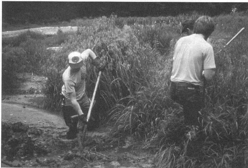
Figure 13. A USBM-constructed wetland for control of metals from acid mine drainage. (USBM photo.)
